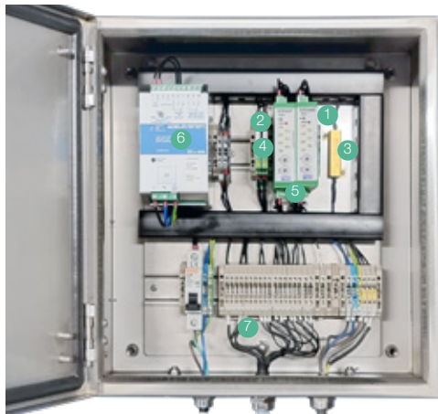
Master unit at the SCADA side
