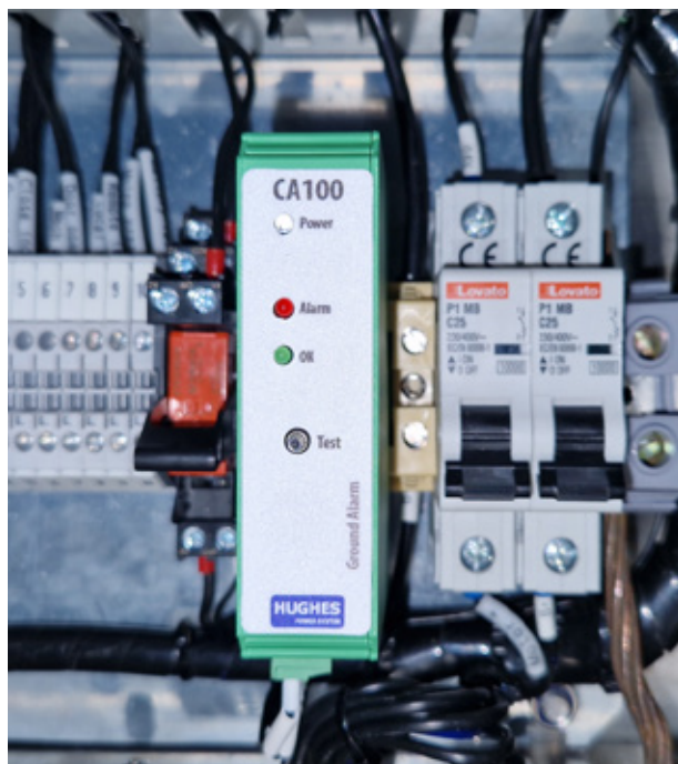
Installation in the motor drive cabinet
